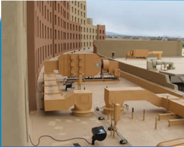
Sandia Resort & Casino installation
